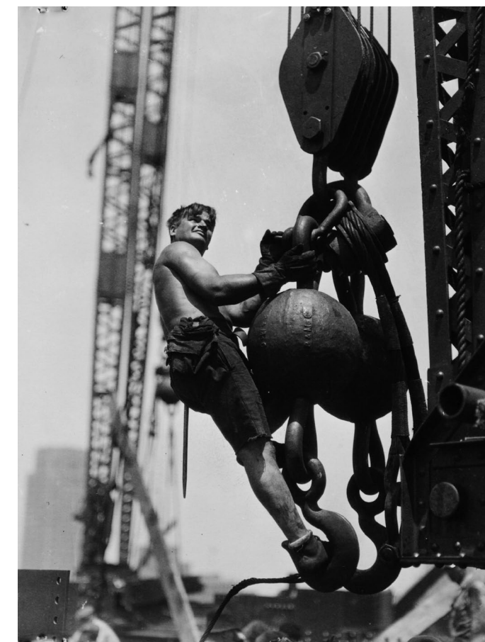
Lewis Wickes Hine, Man on a Hoisting Ball, Empire State Building , 1931. Courtesy of George Eastman House.
