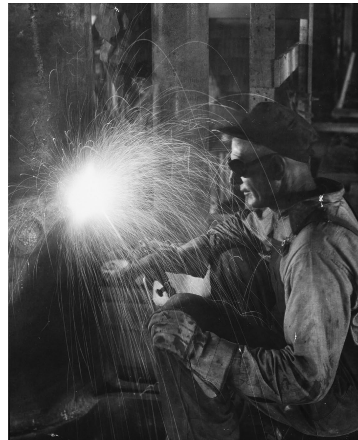
Lewis Wickes Hine, Welder at Work in Empire State Building , ca. 1931. Courtesy of George Eastman House.
